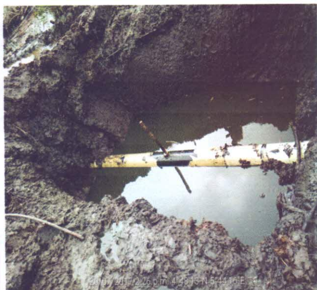
FIG 2: Spill point on excavation
